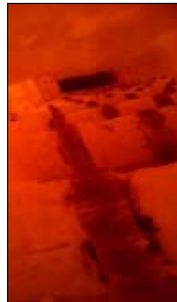
roller hearth furnace
